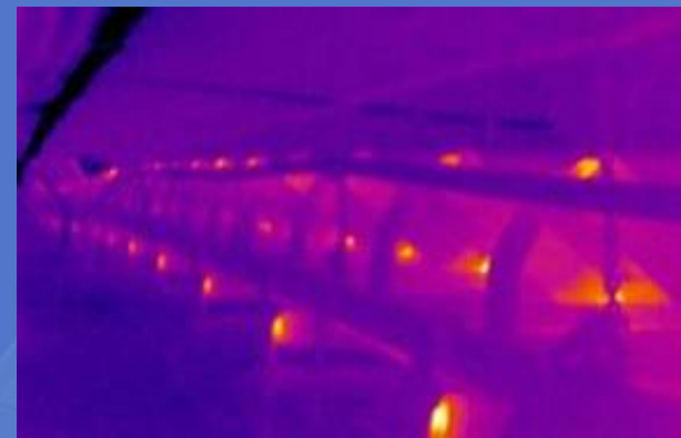
Underground belt line
